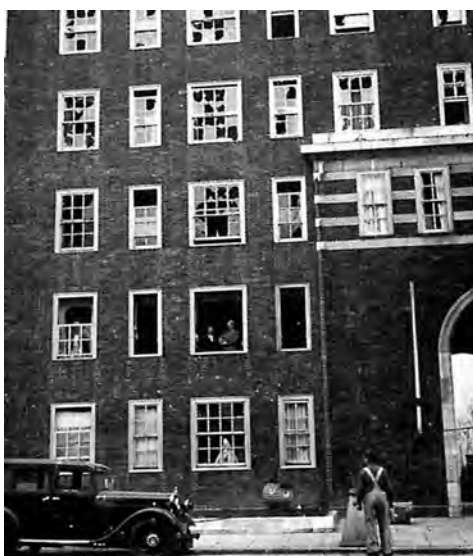
Bomb damage at Raleigh House.
